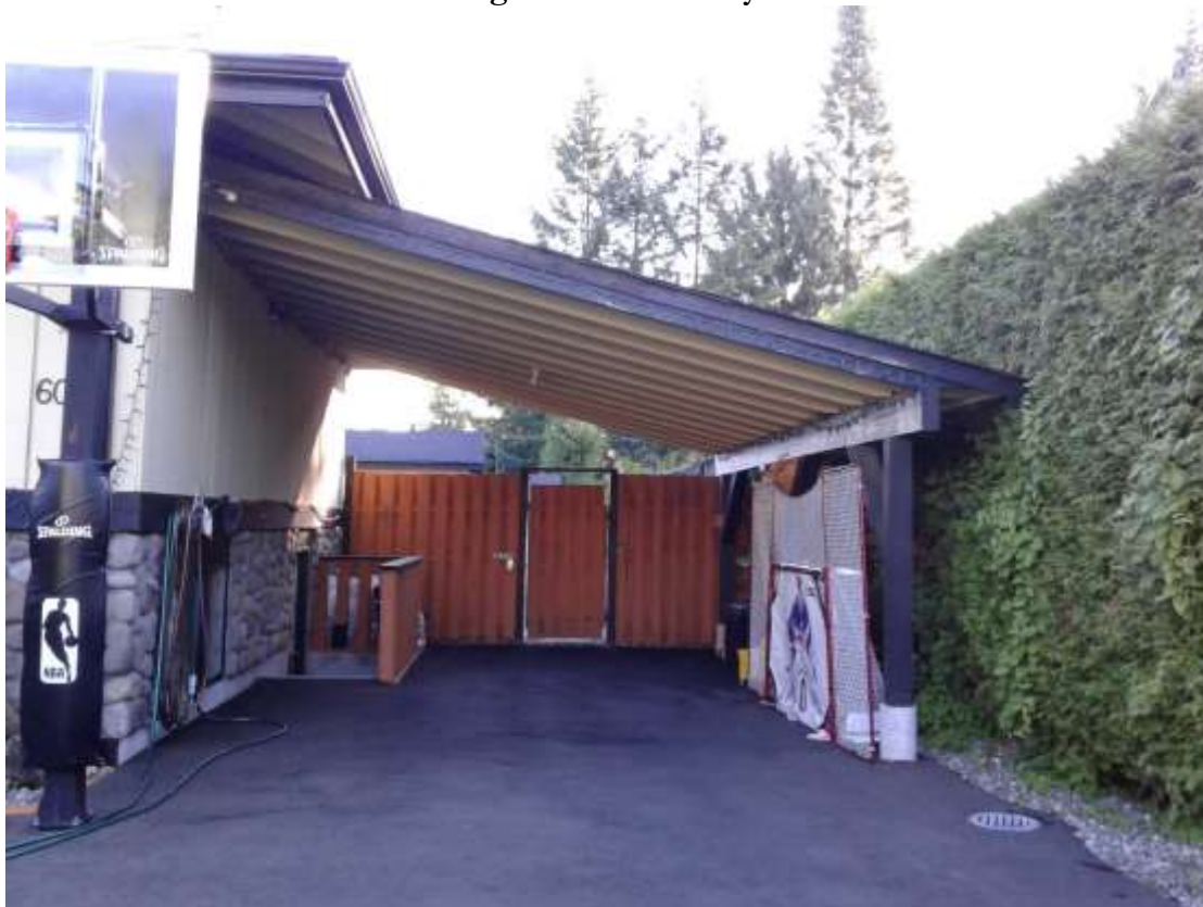
Figure 4: Carport Attached to Dwelling Encroaching Into Side Yard Setback
